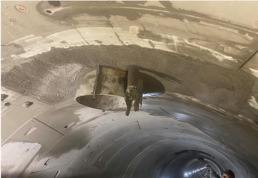
Step 5-6-7: Place three layers of shotcrete on stay-in-place forms. Concrete injection and cut FRP pipe flush to surface of tunnel.
