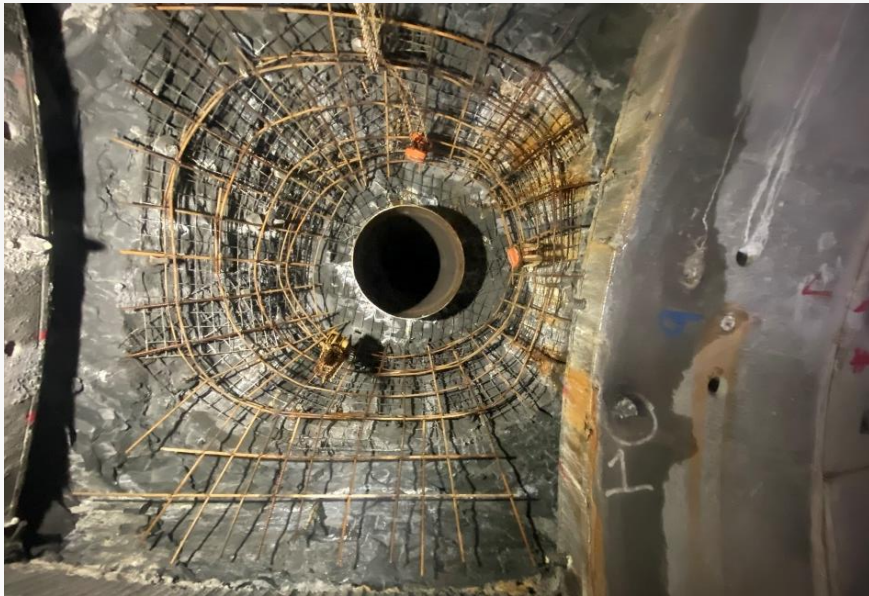
Step 2-3-4: Install rock bolts and wire mesh on rock. Install shotcrete. Drain and remove riser bulkead. Place additional rebar.
